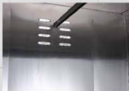
Fresh Air Intake
