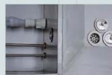
Left Tank Detail
